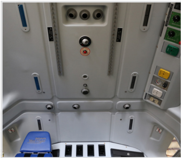
IV Rail and Cabin Lighting
